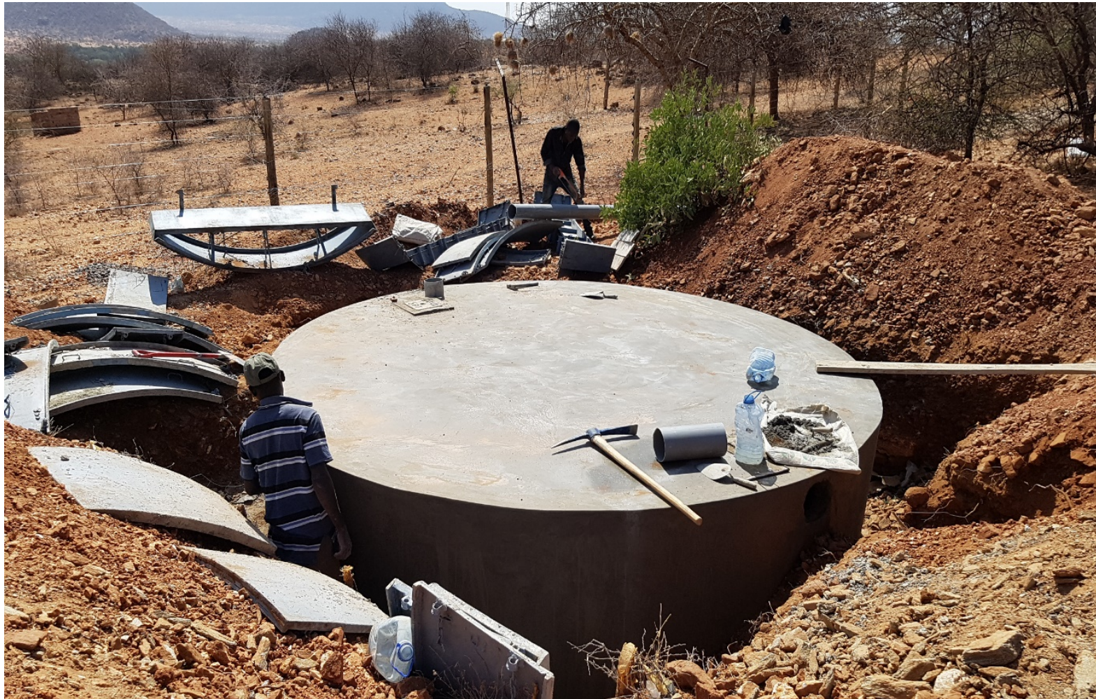
Biologische Septic tank (bio digester)
